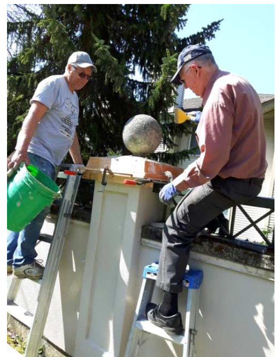
Lloyd Anderson and Barry Miller are seen here rebuilding the base under the ball atop one of our fence pillars. Many of them needed to be repaired. We had a whole crew of volunteers out painting too. What a difference! Thanks guys. (Thanks too, to Zenon Jalbert who sent me this picture.)
